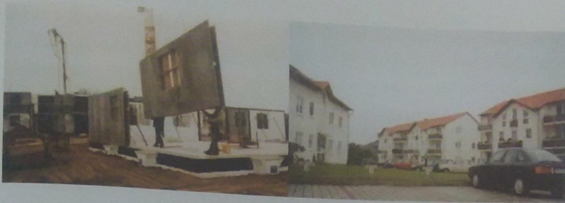
Fig.8. Complex of apartments in Osterweddingen under construction and Fig.9. Complex of apartments in Osterweddingen build with the DUO-MASSIV system (Van elten, 2006).
