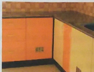
Fig: Side cabinet
