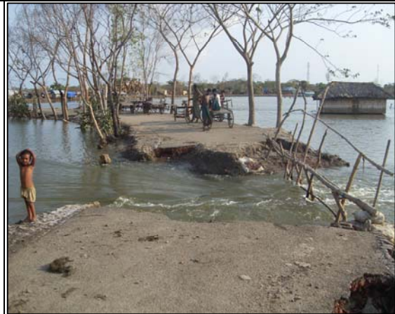
Roads are destroyed by Aila at many places in Koyra UZ, making SRF actors more vulnerable- needs serious rehabilitation.
